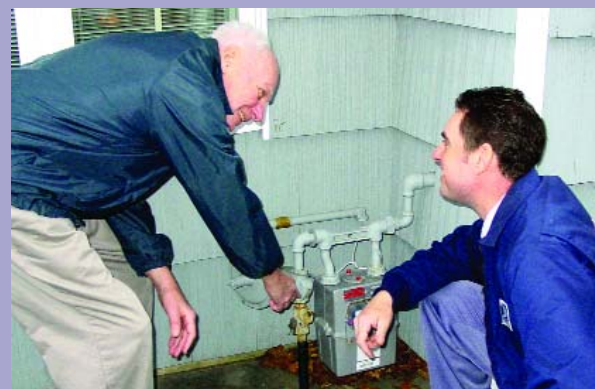
L.I. Mgd., NY Branch 6000 member Anthony Villani (r) and patron Thomas Fisher revisit the site of a gas leak detected by the carrier.
